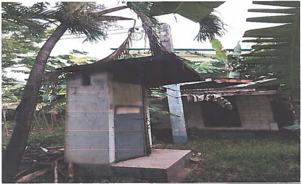
Electrical Breaker Closet
