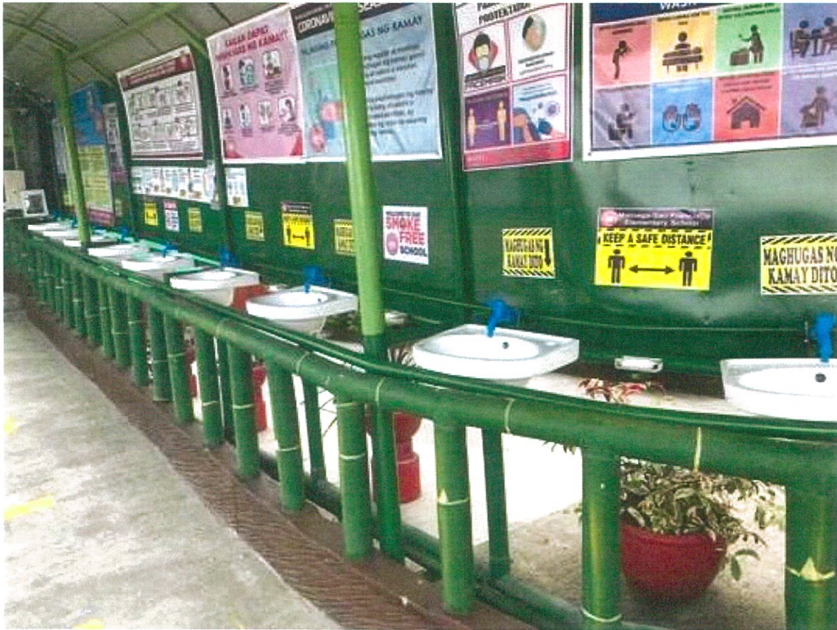
Handwashing facilities for school children of Mainaga-San Francisco Elementary School
