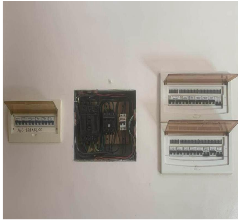
Existing panel board and circuit breakers - 1 lot
