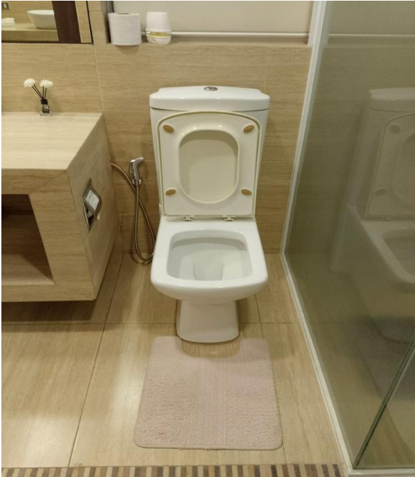
Existing Water Closet – 5 sets
