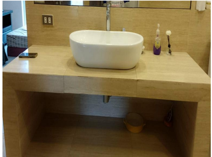
Existing Wash Basin – 5 sets
